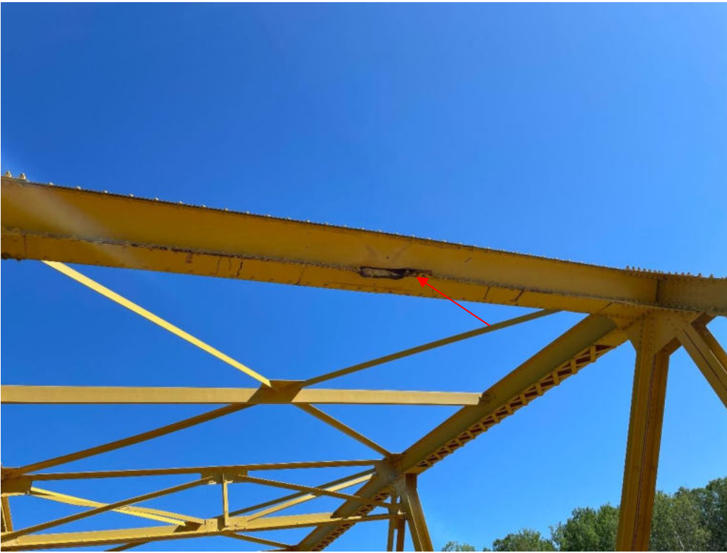
5. S6 -U9U9 damaged
