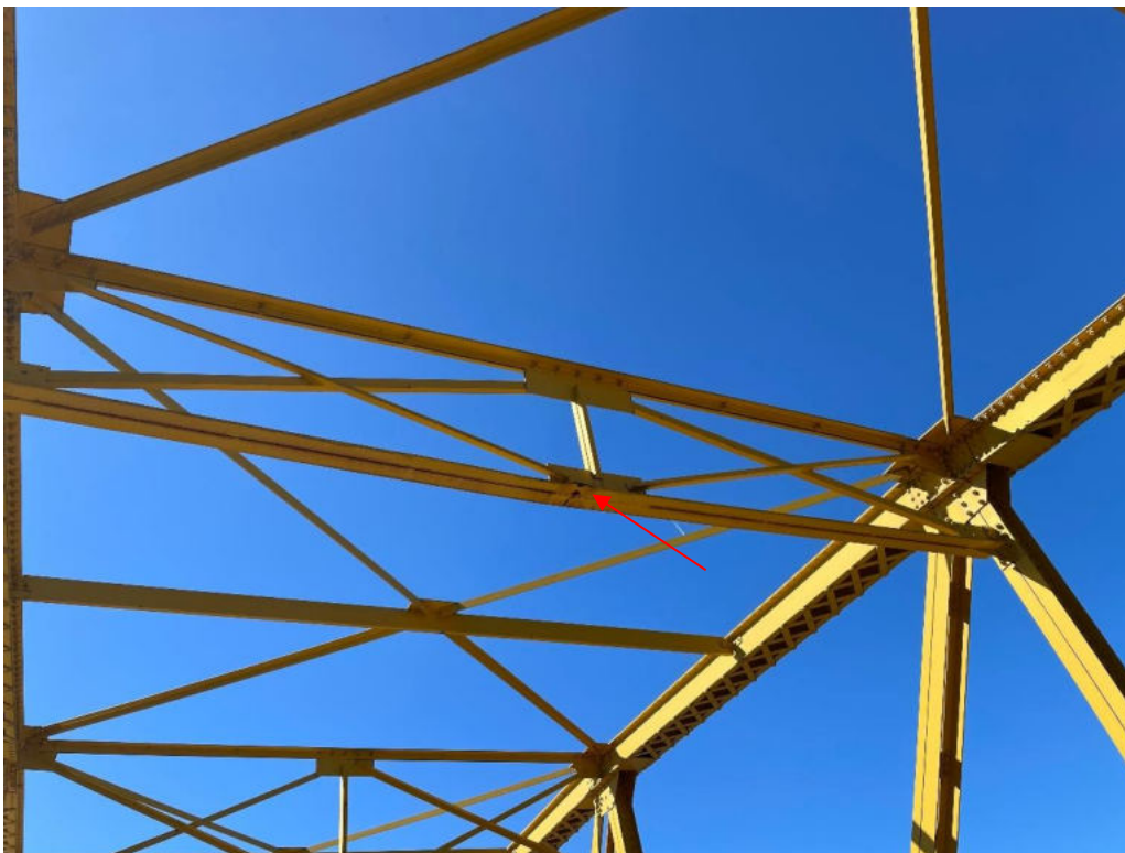
2. S6 - U2U2 damaged
