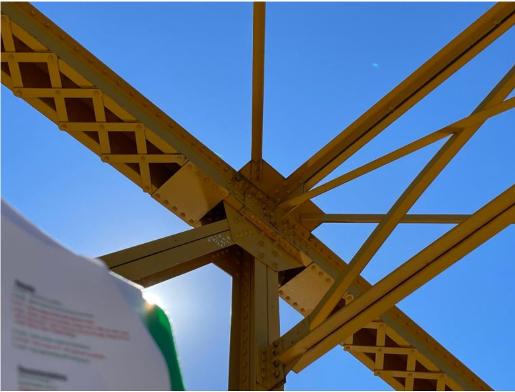
15. S4 - L6U7 E damaged
