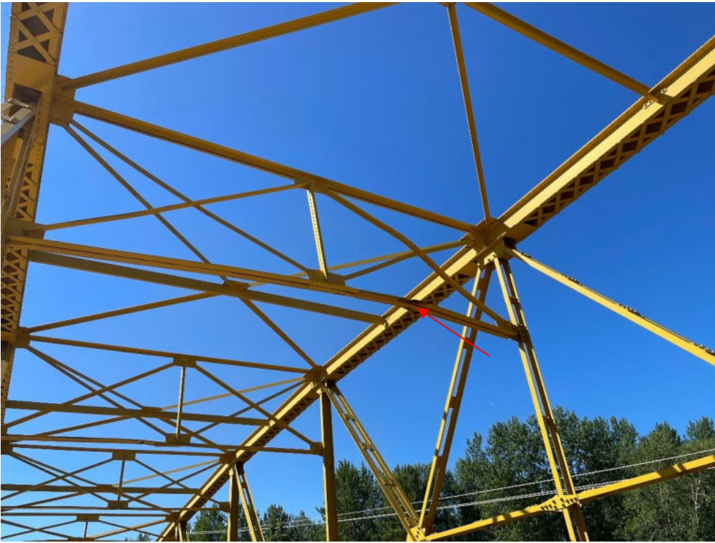
13. S4 - U5U5 damaged
