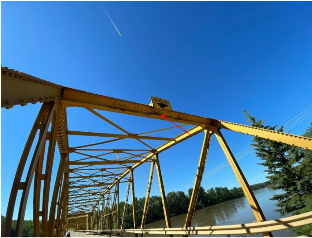
1. S6 - U1U1 damaged
