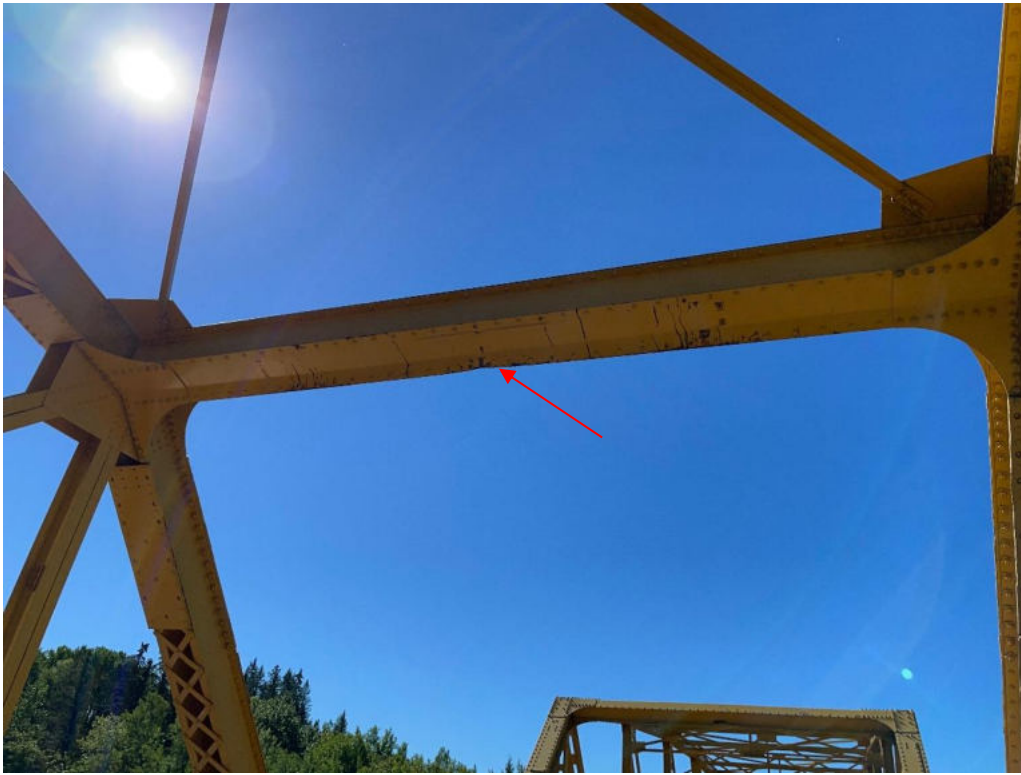
9. S5 - U11U11 E damaged
