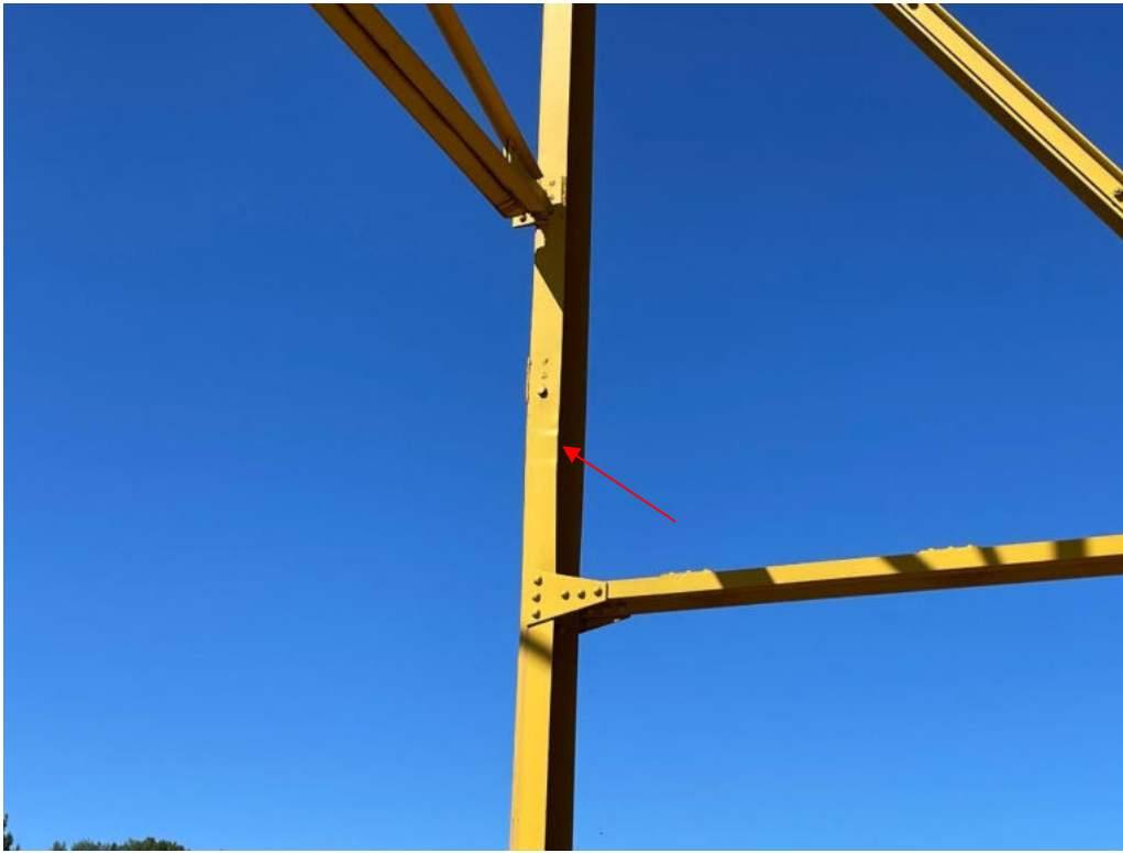
11. S5 - L9U9 damaged
