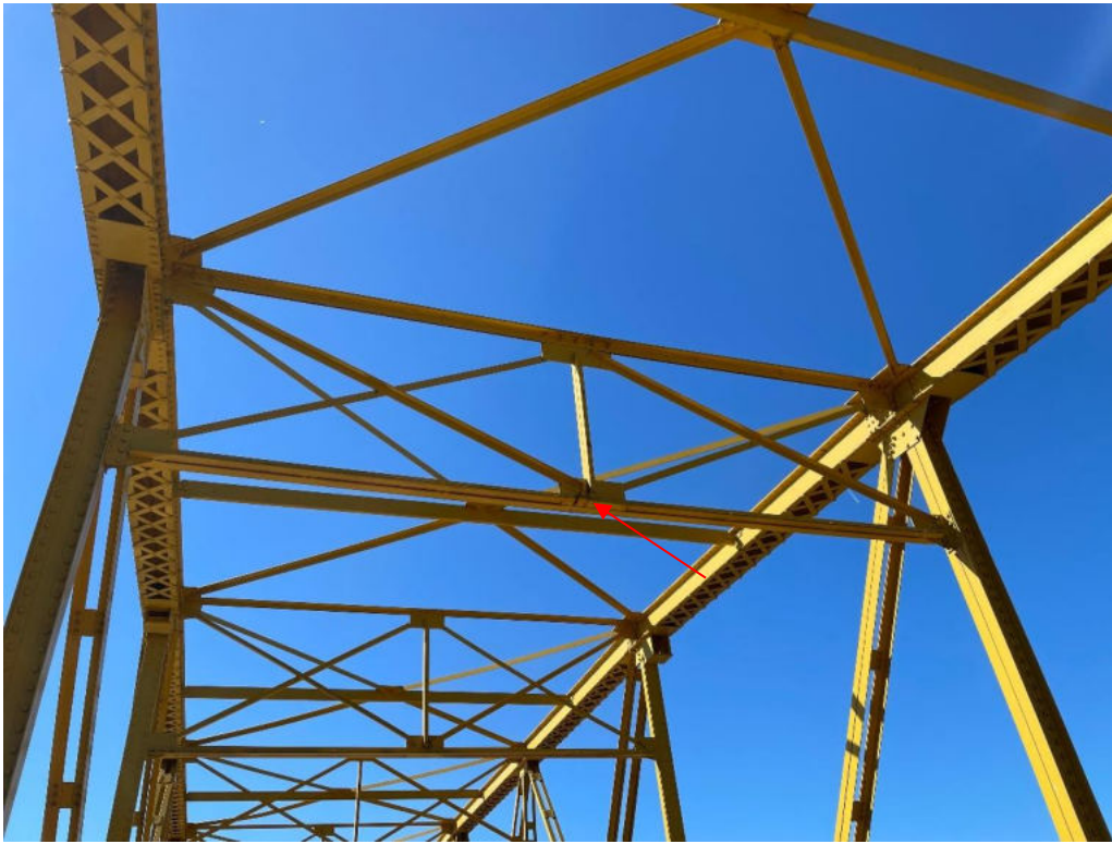
3. S6 - U3U3 damaged
