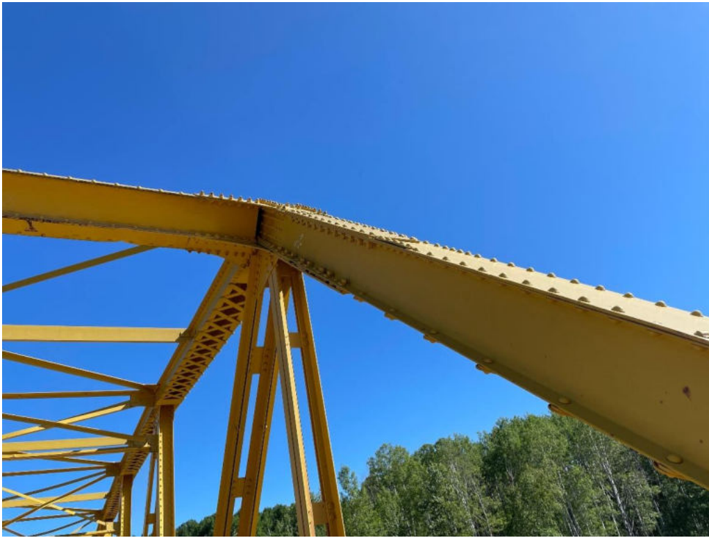
7. S6 - U9L10 E damaged
