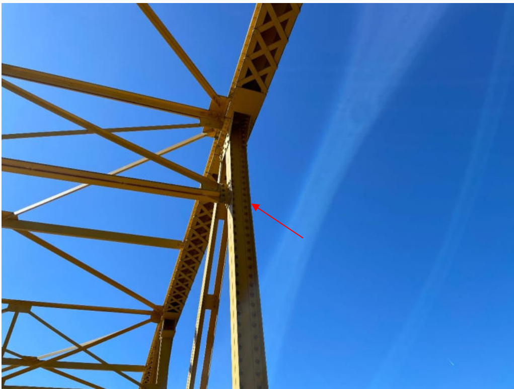
4. S6 - L3U3 damaged
