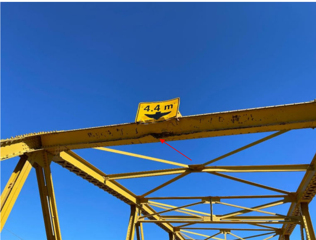
16. S4 - U9U9 damaged
