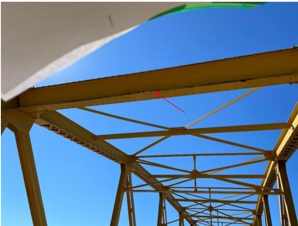
8. S5 - U1U1 E damaged
