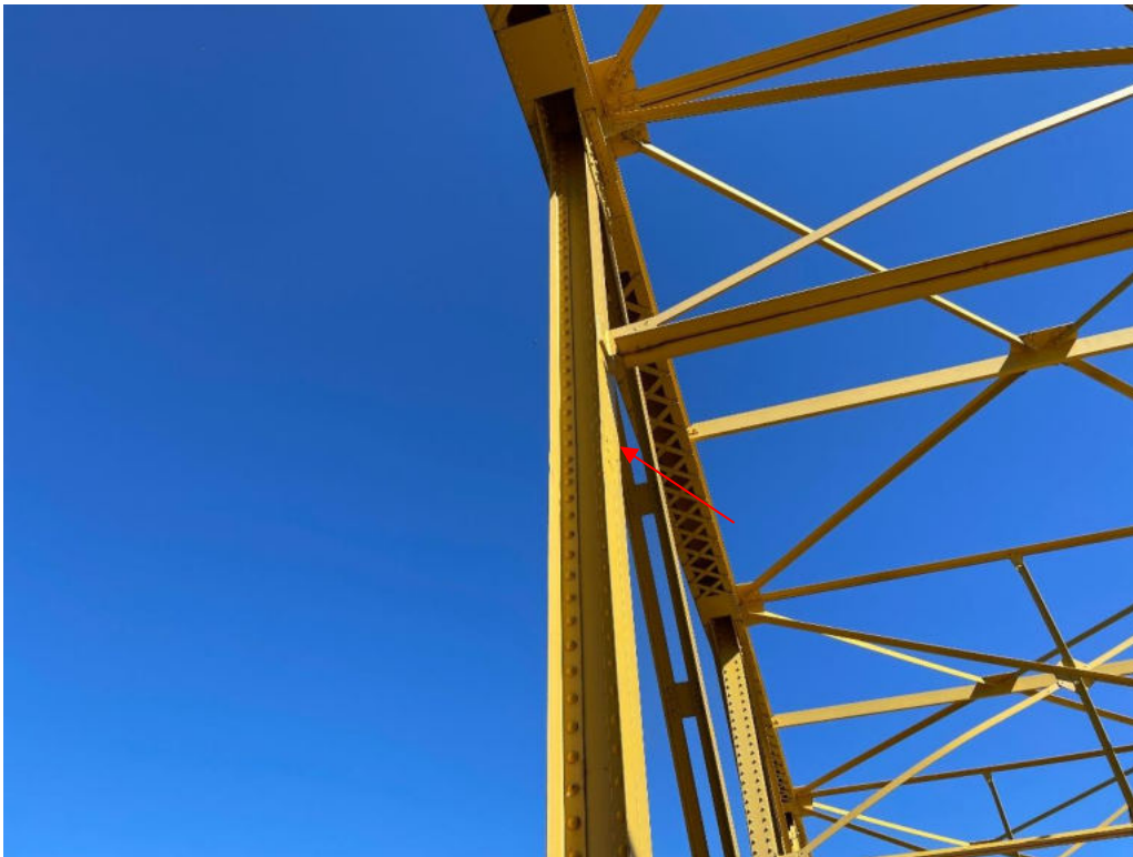
10. S5 - L8U8 damaged
