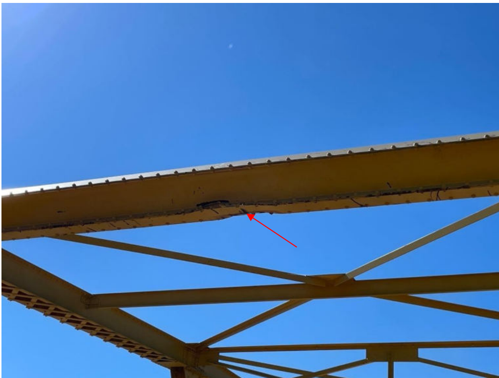
12. S4 - U1U1 damaged
