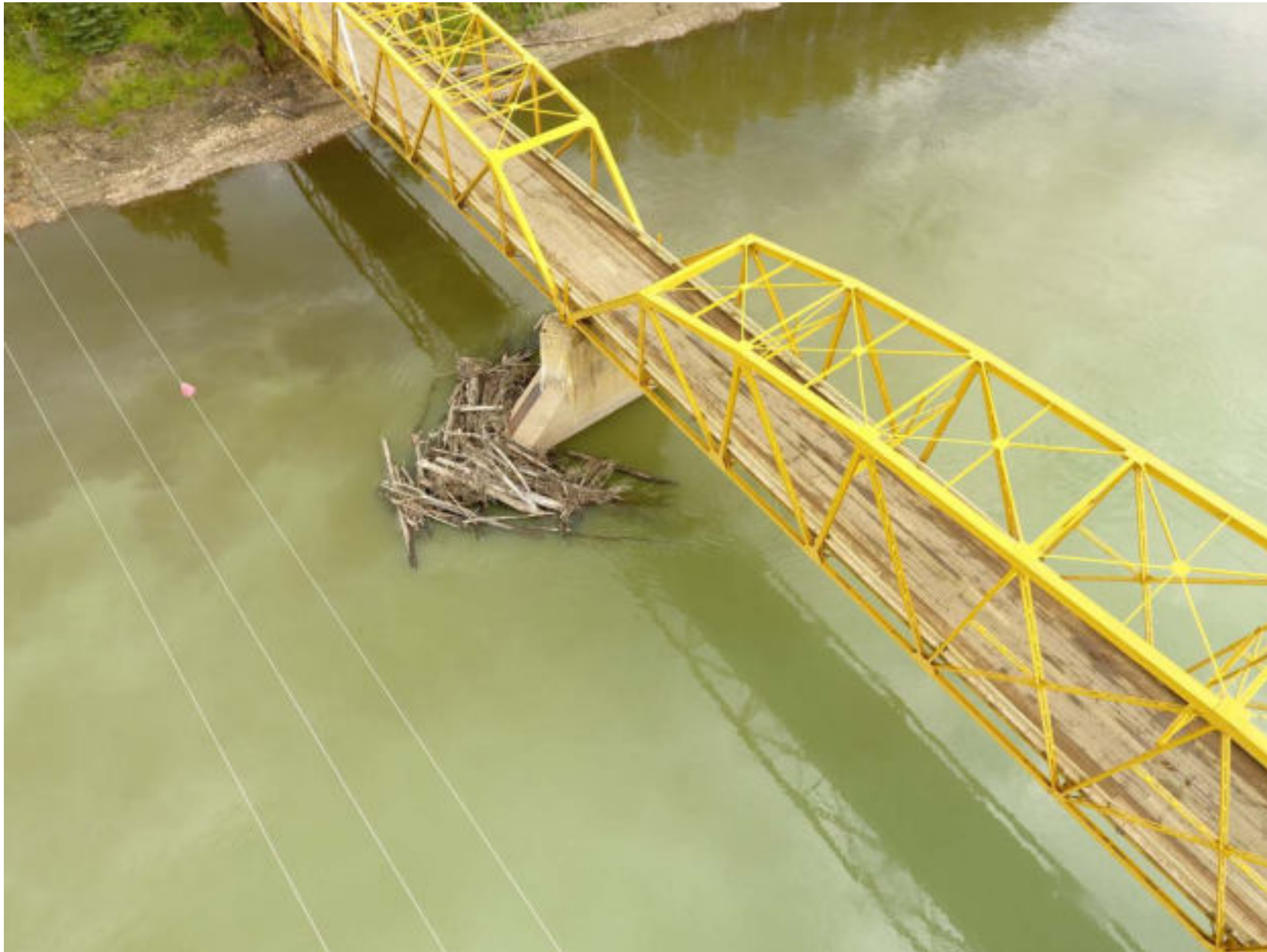
Site Photo 7 – Drifts at Pier 3
