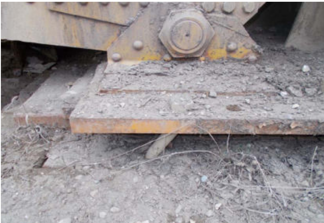
38. One A/B at P6 east bearing bent. Possibly due to north hill and P6 moving towards river
